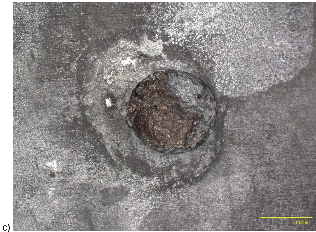
Figure 5 (cont.): c) lower hole – blocked.
