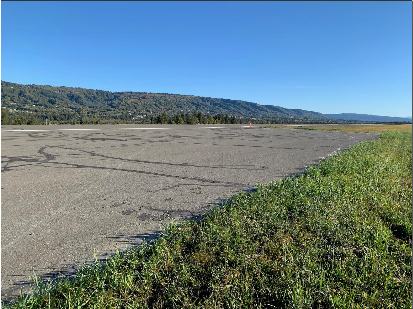
Photo 2 – Accident site, view from near the accident site to the approach end of the runway.
