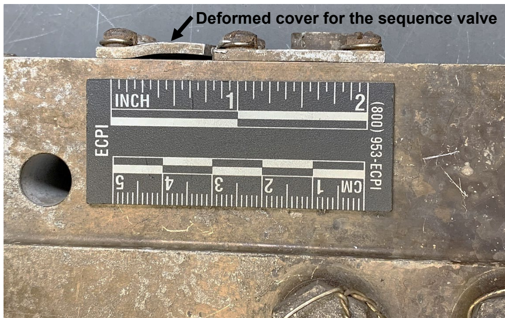
Appendix 2B. Side view of the deformed cover for the internal sequence valve.
