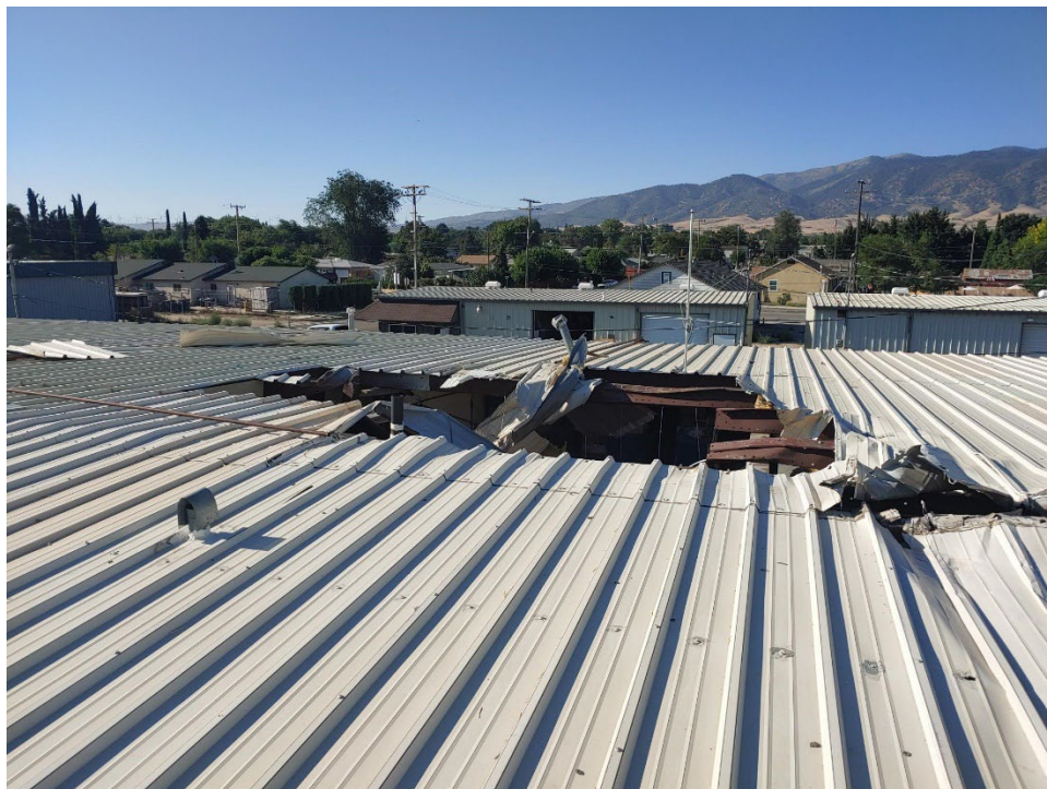
Figure 6: Roof Damage (Post Airplane Recovery)
