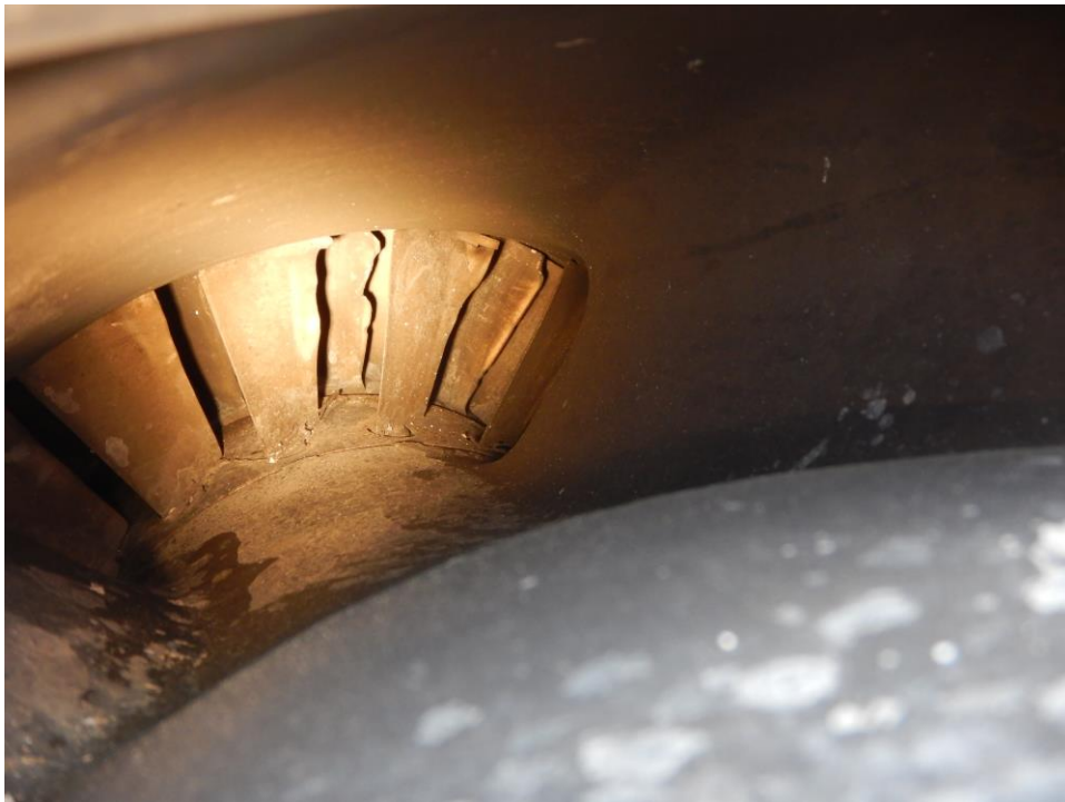
Figure 32. IGV and Compressor Damage
