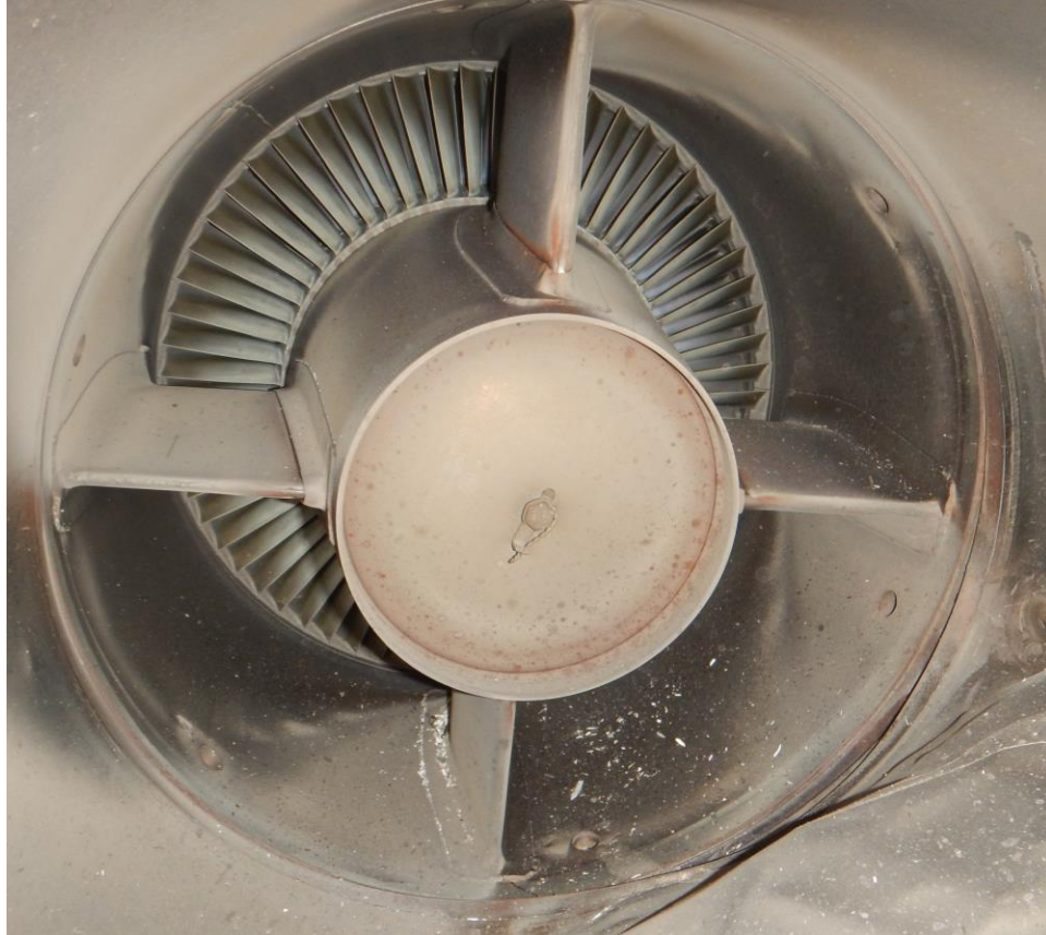
Figure 33. No Visible Damage to 2nd Stage Power Turbine Blades or Stator Vanes
