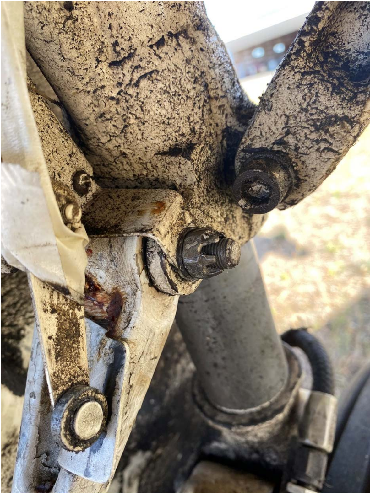
Missing Cotter pins
