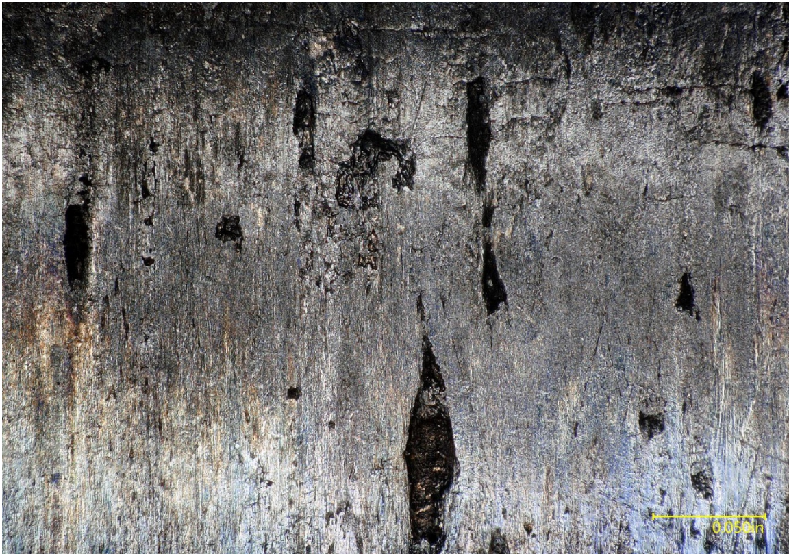
Figure 27 – Closer view of the spalled material on the inner surface of the C4 cap remnant.
