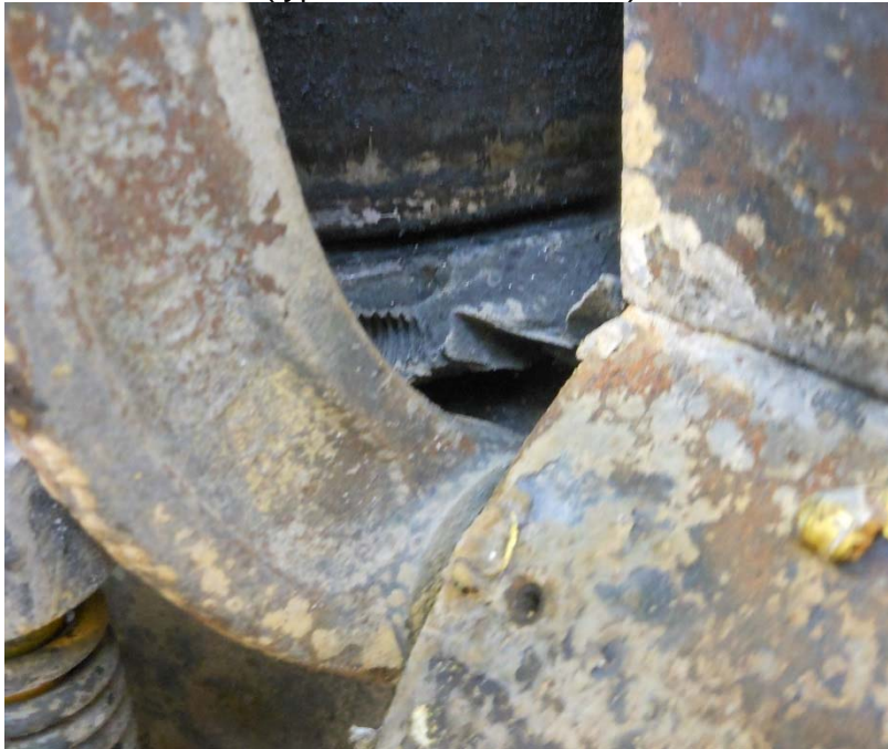
Photo #11 - Right prop gouge in guide collar (typical all three locations)
