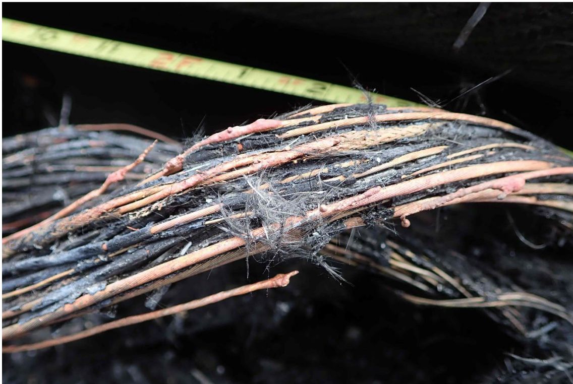
Figure 8 – Arcing Damage at Station 120
