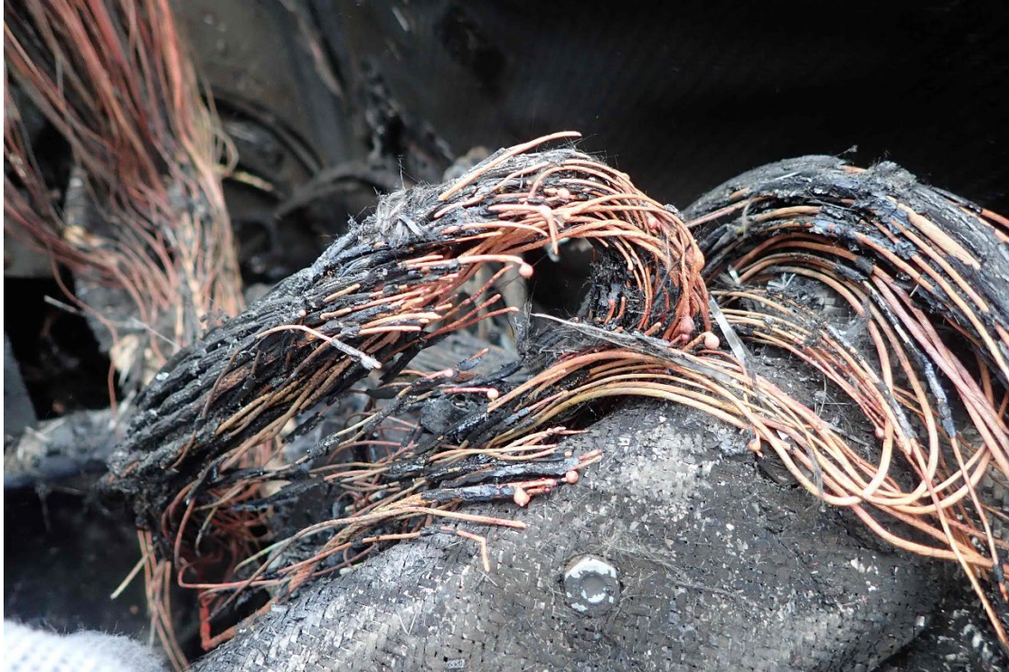
Figure 7 – Arcing Damage at Forward Grounding Block at Station 113
