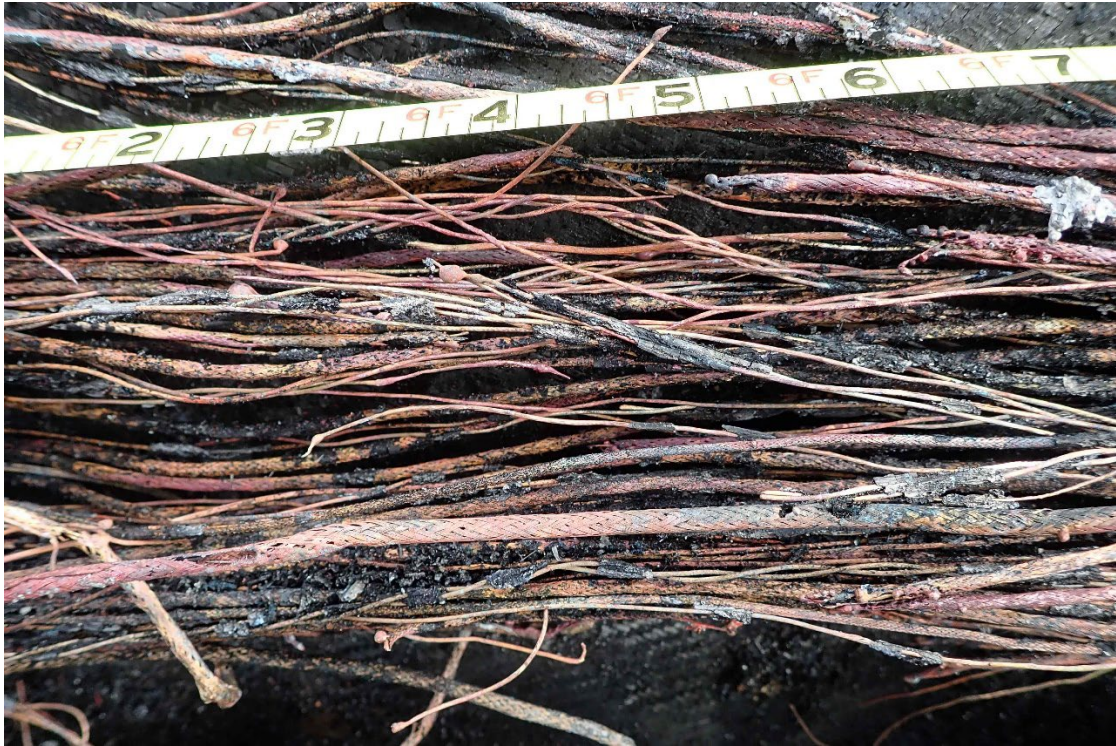
Figure 9 – Close Image of Arcing Damage in General Area Between Station 151 through 179
