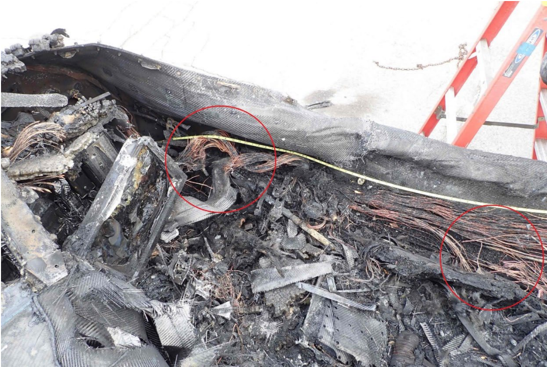
Figure 5 – Arcing Damage at Forward Grounding Block at Station 113
