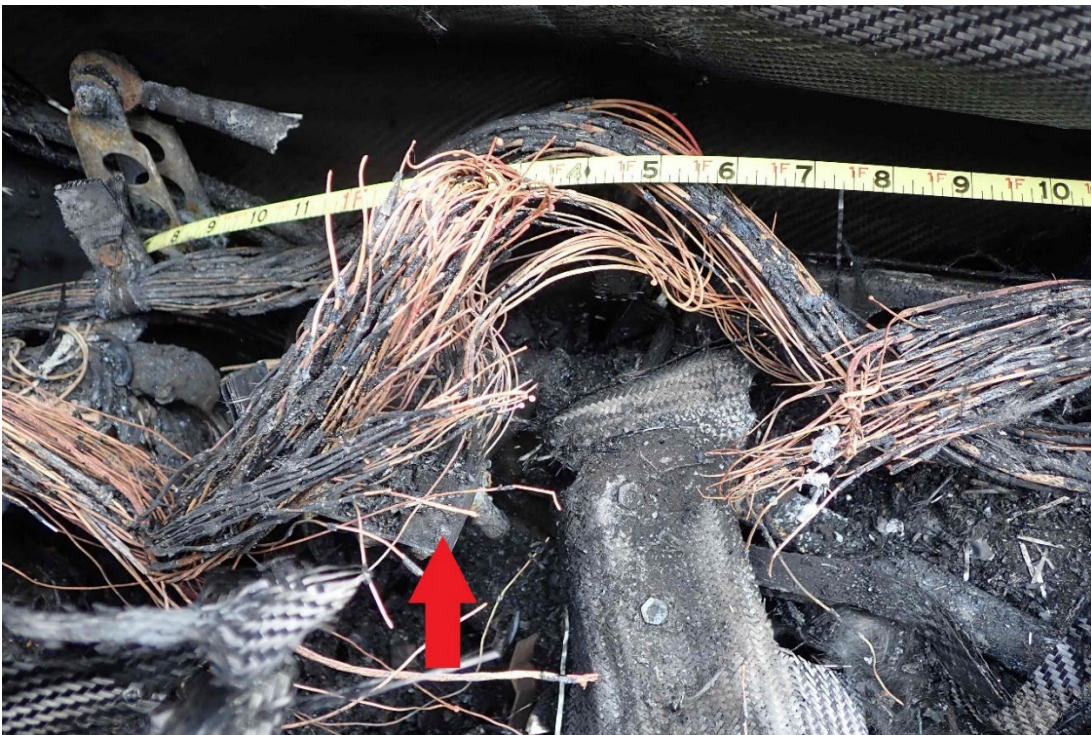
Figure 6 – Arcing Damage at Forward Grounding Block at Station 113 (block indicated by red arrow)
