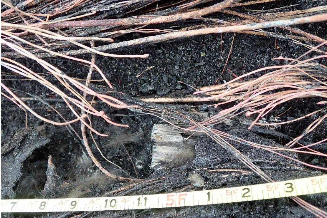
Figure 11 – Arcing Damage in General Area Between Station 151 through 179
