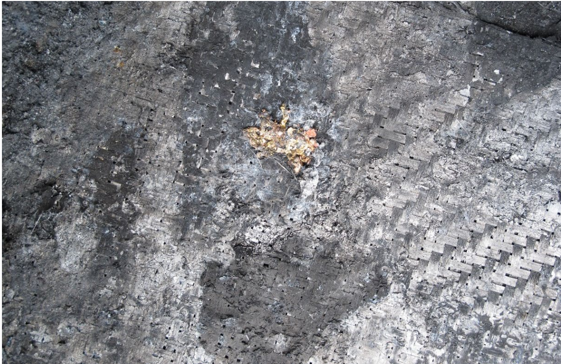
Figure 13. Close-up photograph of copper-colored deposit on right sidewall.
