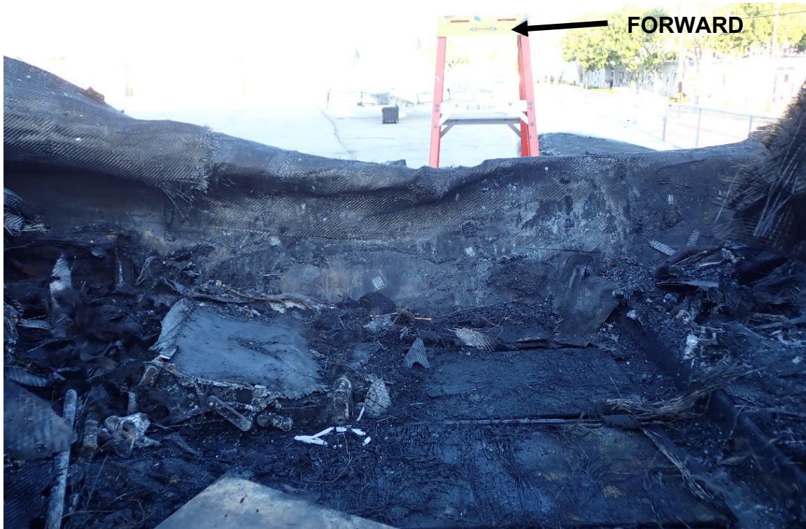
Figure 3. Floor area after debris removal.
