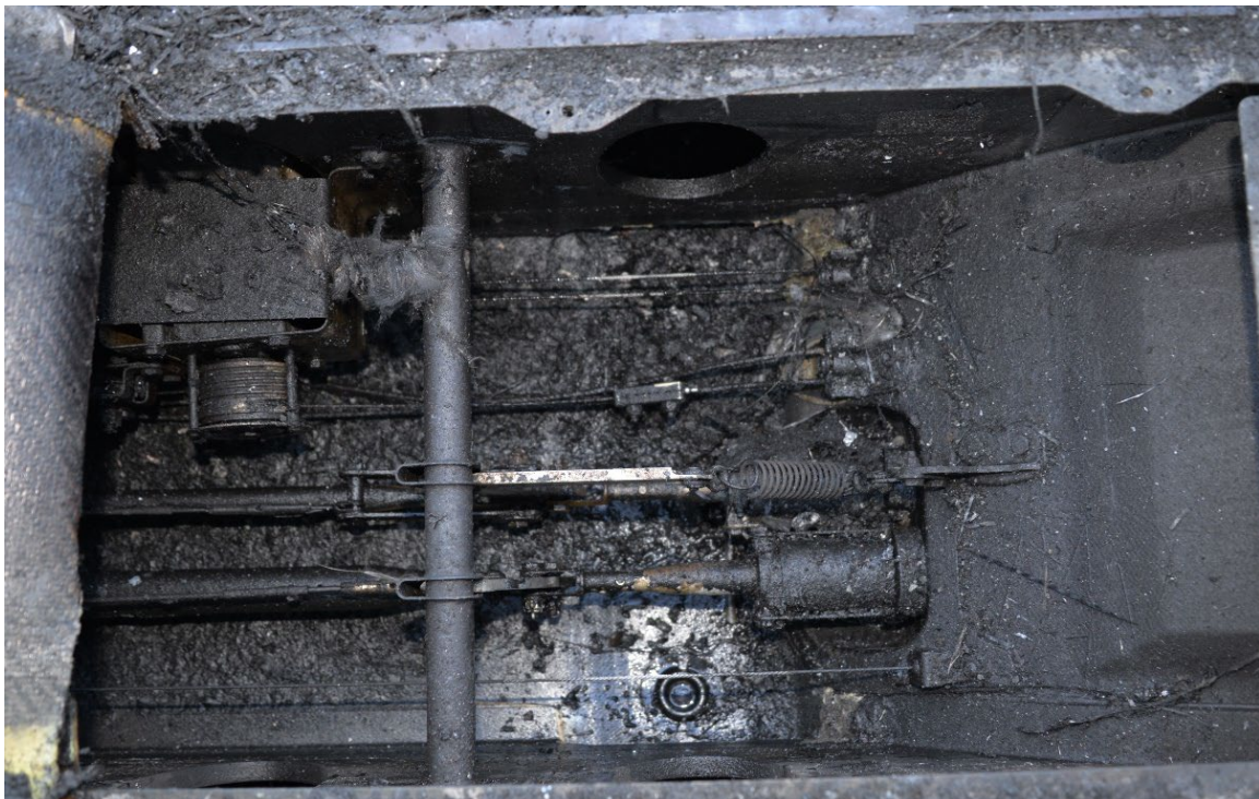
Figure 6. Servo located centerline under floorboards.
