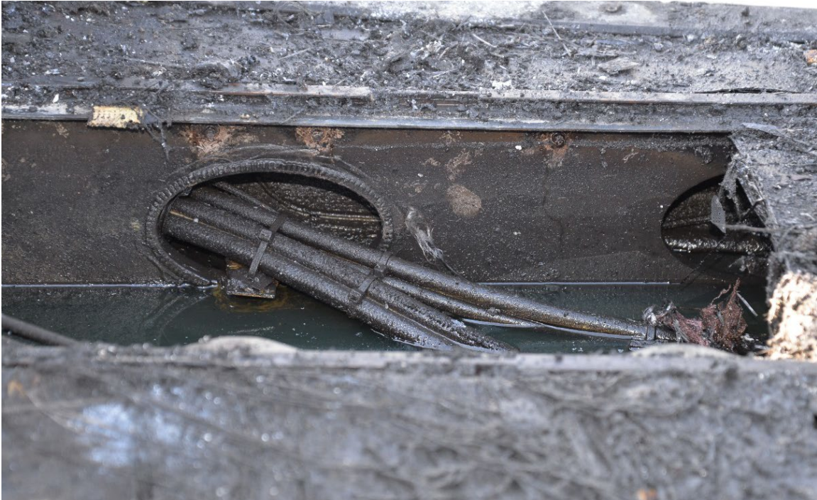
Figure 7. Wiring under left side floorboard.
