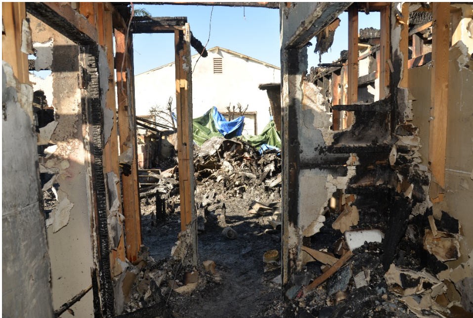
Figure 2: Overview of Main Wreckage from Adjacent Room
