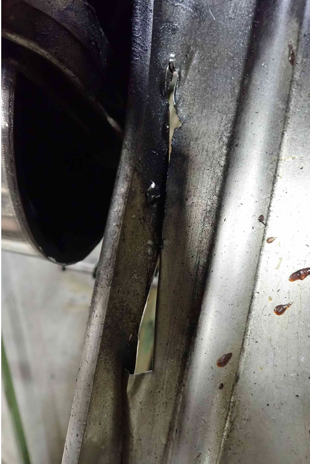
Photo 9 – Cooling Fan Shroud
