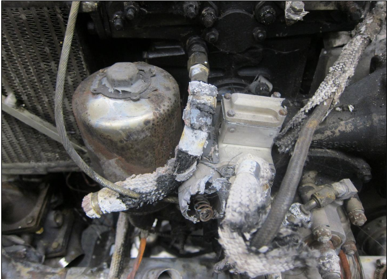
Figure 6-Engine driven fuel pump installed on the engine.
