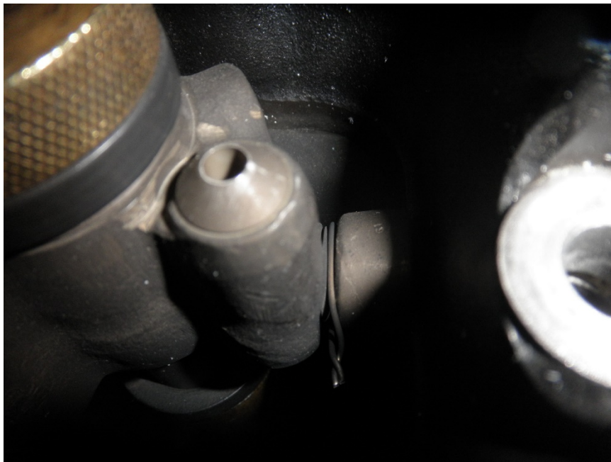
Photo No. 10: Close up view of loop of safety wire around end of boost rack.
