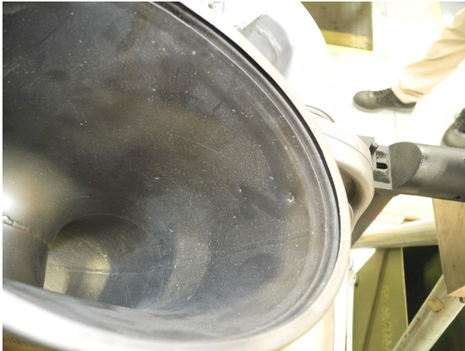
Photo 2 – Exhaust Duct – Small Dents
