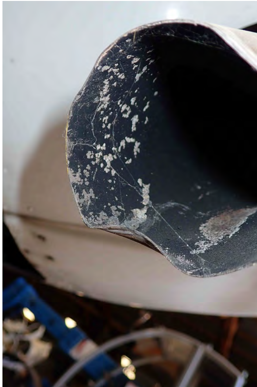
Photo 2 – Inner Surface of Exhaust Pipe
