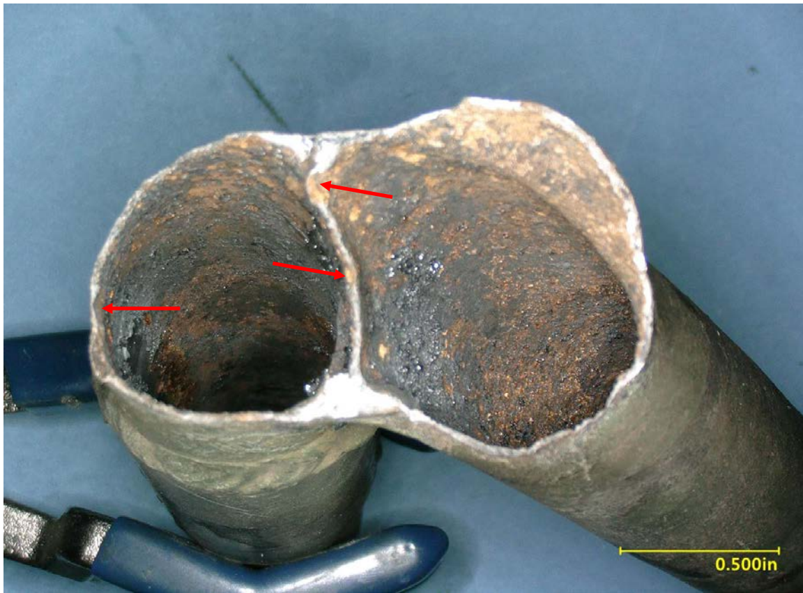
Figure 10: Digital microscope image showing corrosion deposits on the internal surfaces of truss tubes II and III. The red arrows indicate wall thinning due to corrosion.
