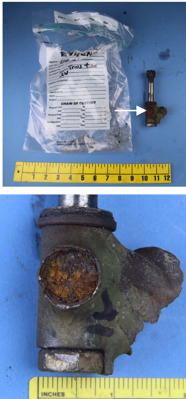
Figure 3: The top photo shows an overall view of truss tube IV. The white arrow points to the viewing perspective in the close-up shown in the bottom photo.
