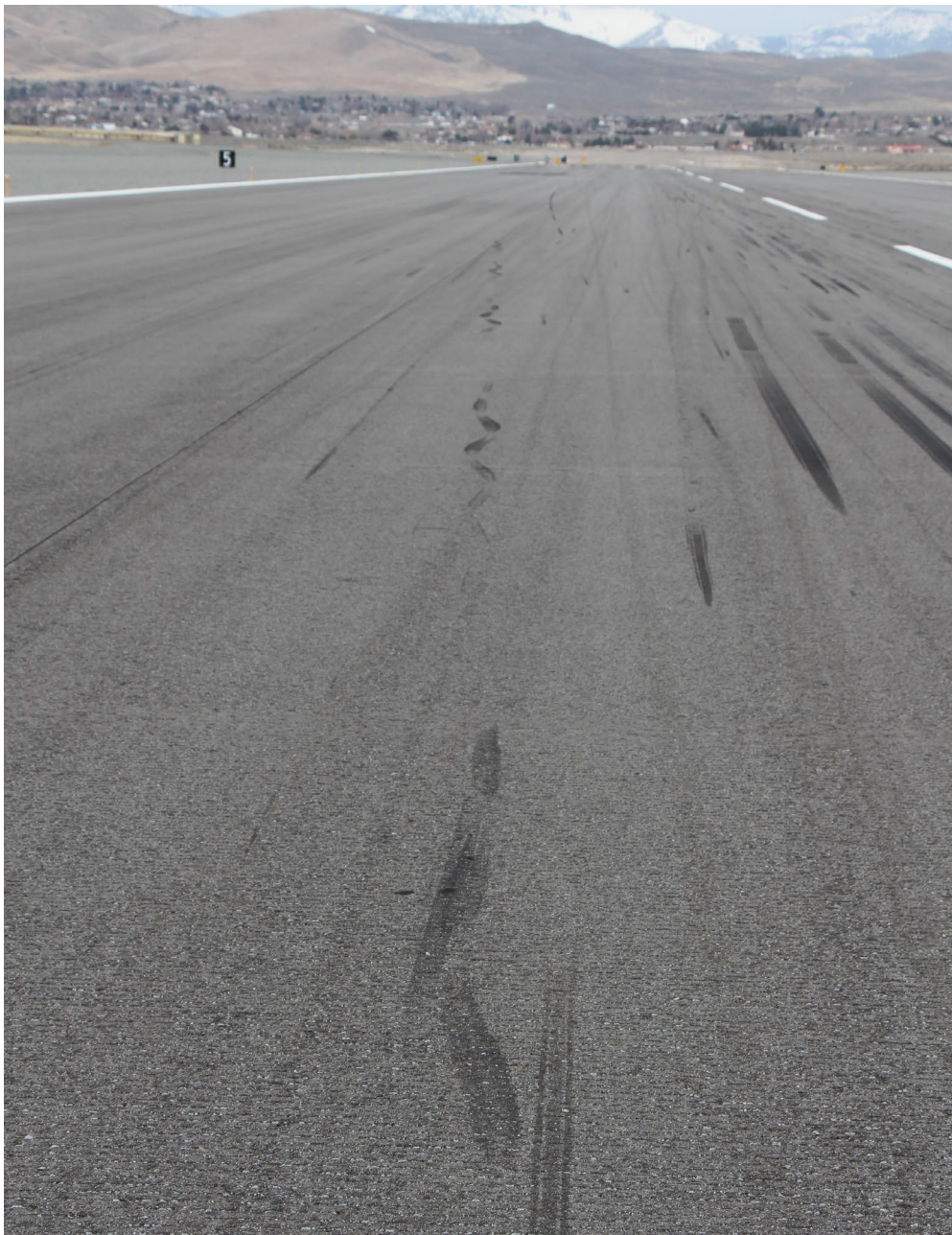
Photo 3 – Tire Marks on Runway from Accident Airplane (Courtesy of Airport Manager)
