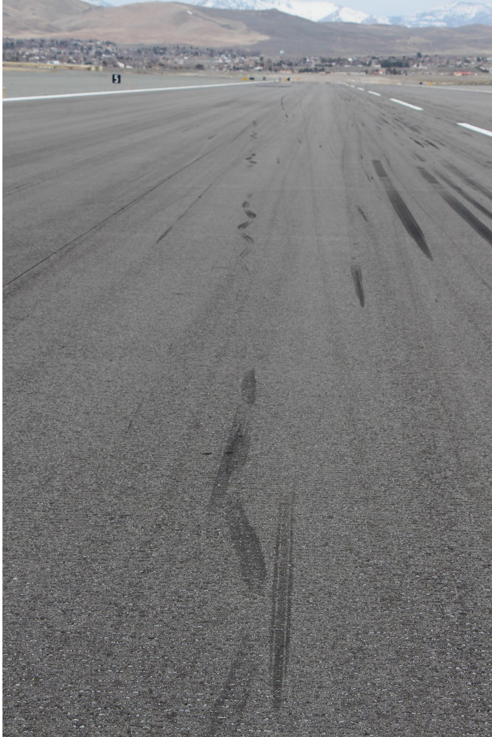
Photograph 2: Tread Marks on Runway Originating at Taxiway B (Airport Manager)
