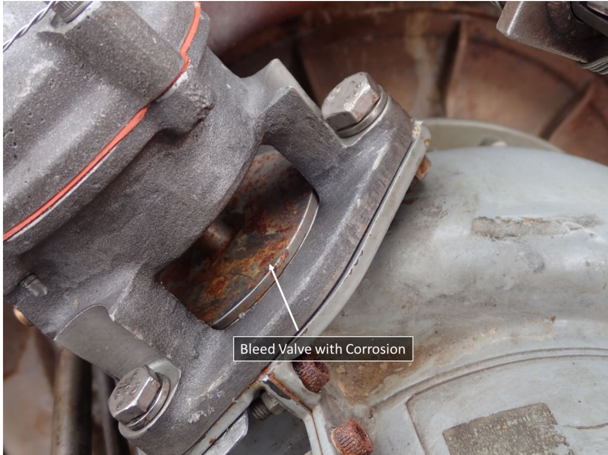
Figure 10. View of the compressor bleed valve, showing corrosion on the valve. Photo courtesy of Rolls-Royce.
