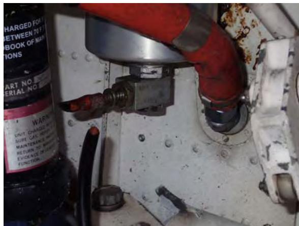
Airframe Fuel Filter Return
