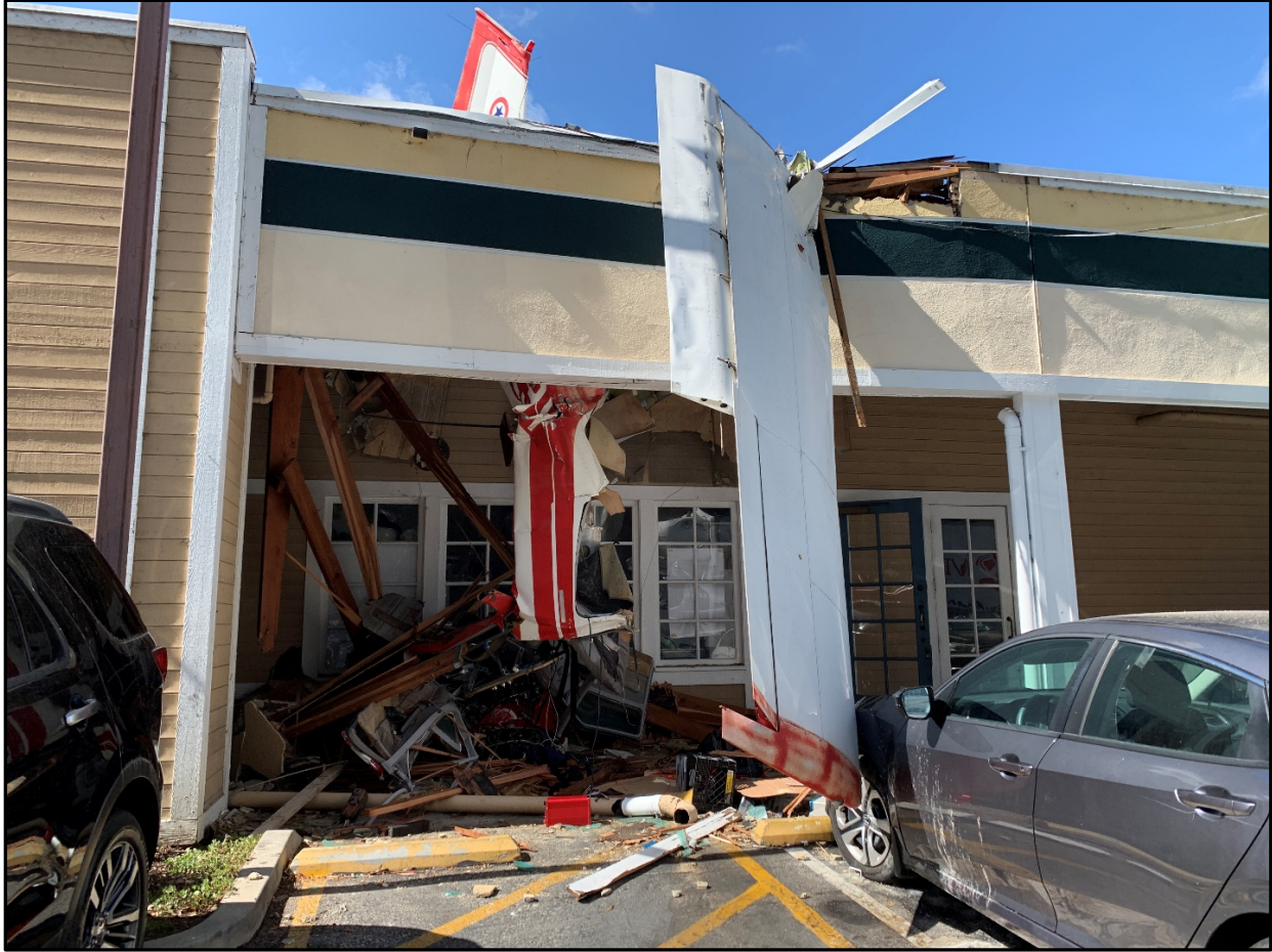
Figure 2: Airplane wreckage as viewed from the ground.
