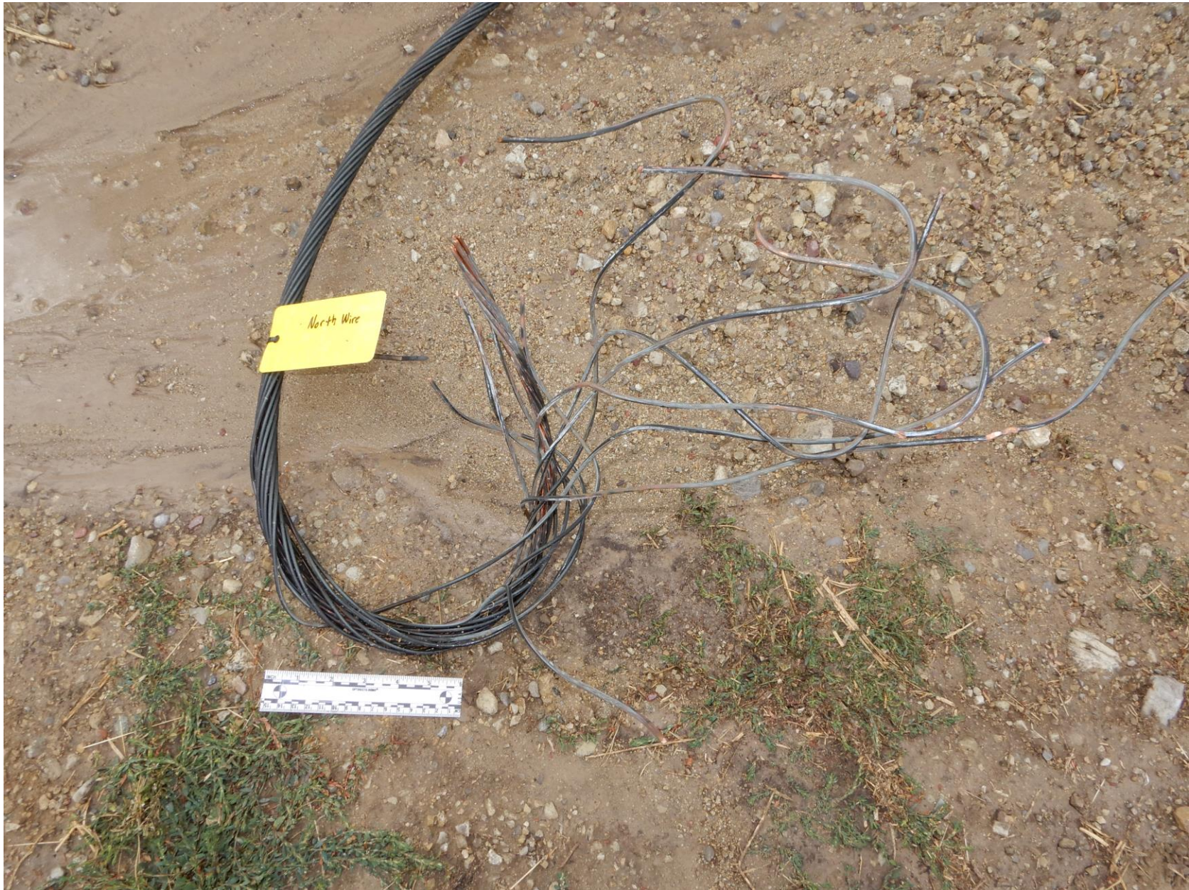
Photo 13. Eastern most power distribution line, north side
