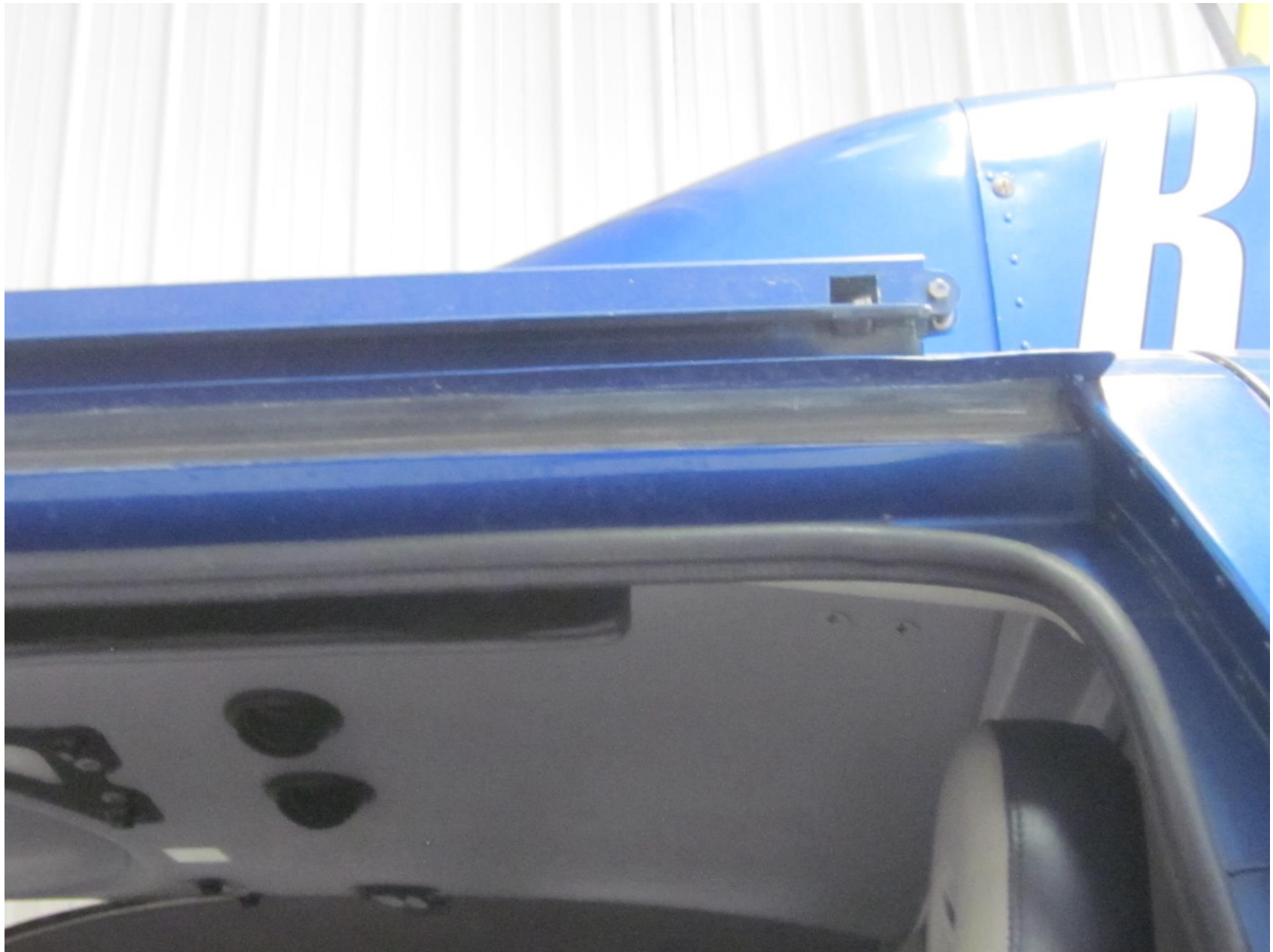
Photo 3 – Left Side Sliding Door Upper Track
