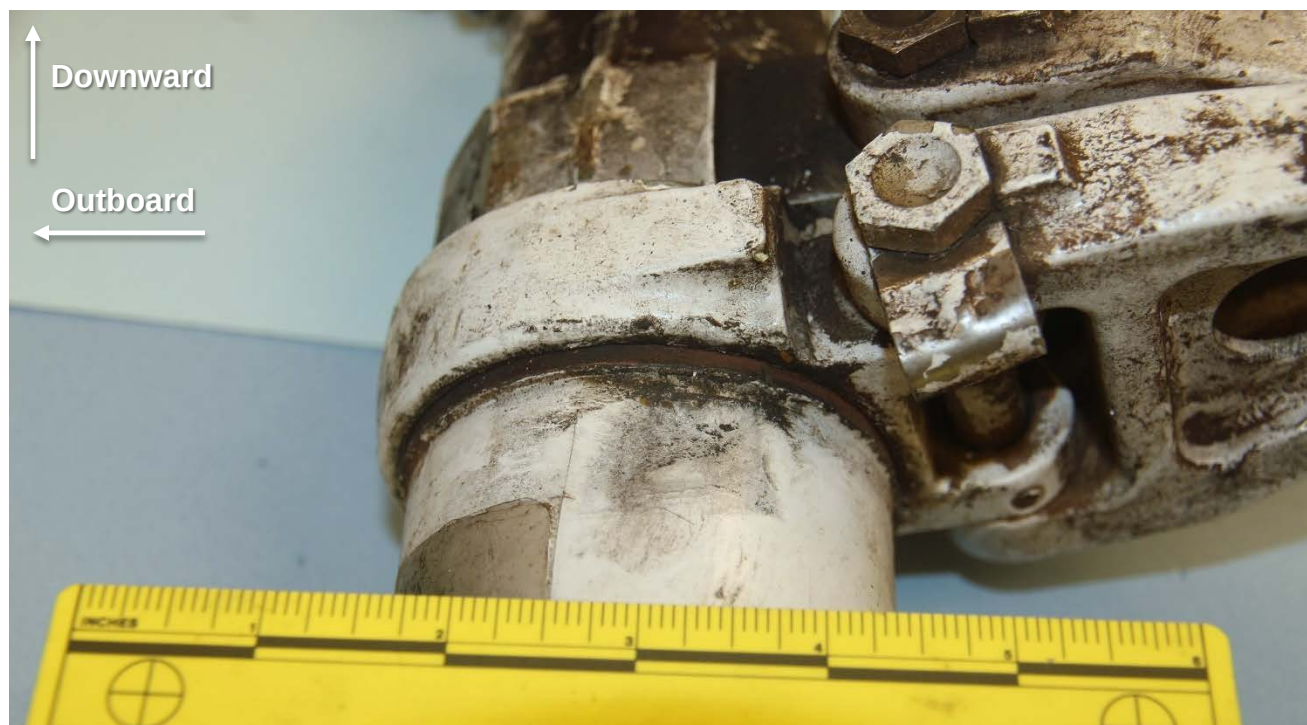
Figure 3 – View of the loose attachment joint, looking downward, showing the gap consistent with a fractured weld.
