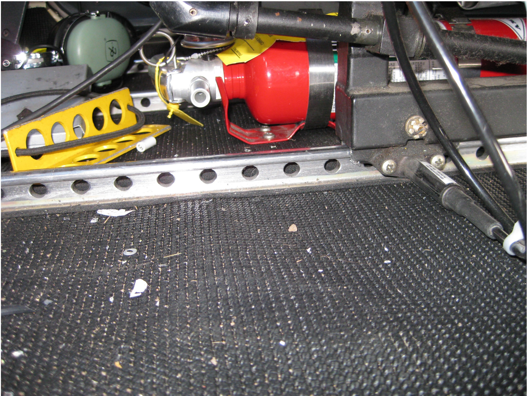
Photo 3 – Seat Rail (Photo Courtesy of the FAA)
