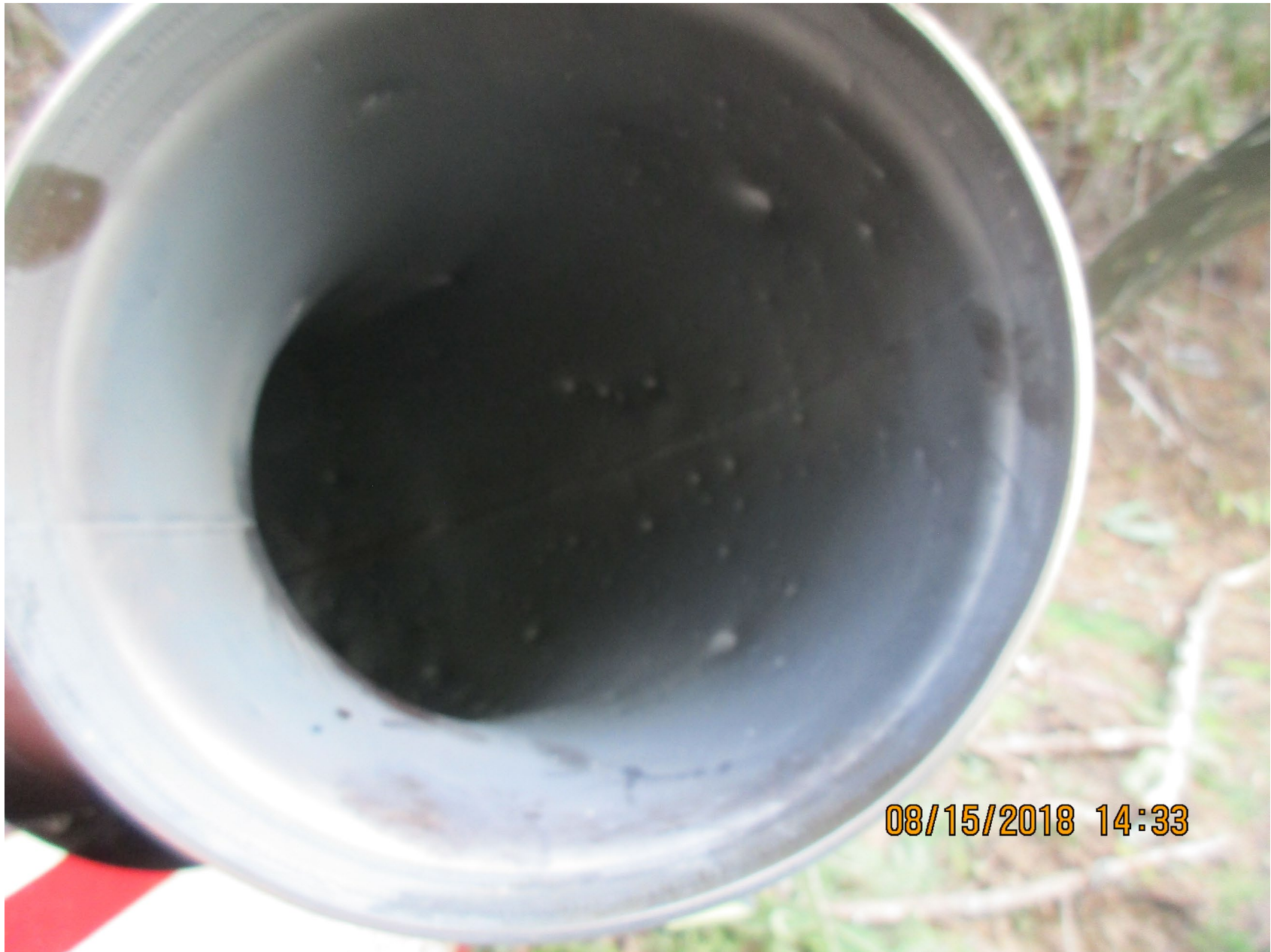
Photo 4 – Exhaust (Photo Courtesy of FAA)
