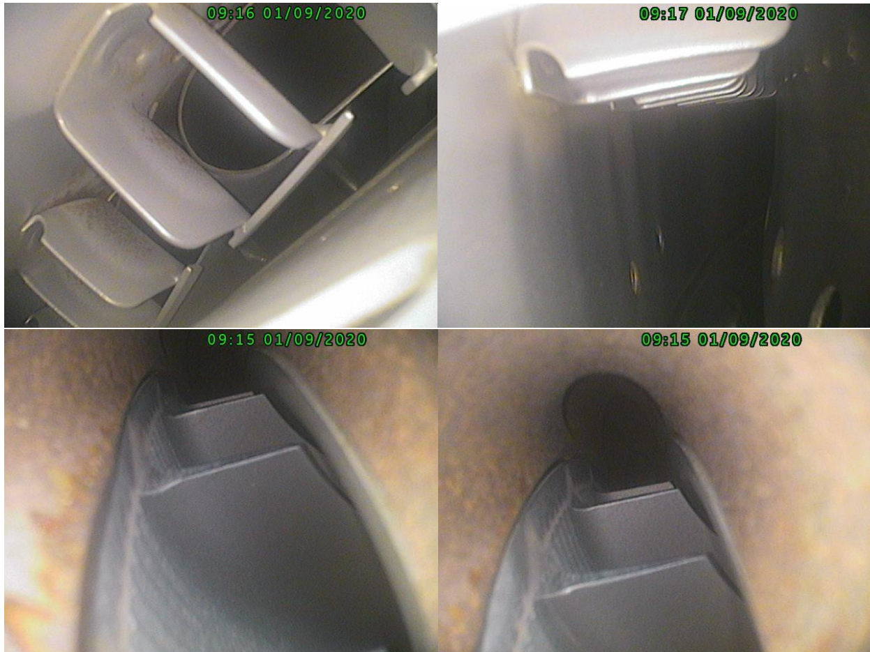
Photo No. 4 Diffusers area and centrifugal compressor
