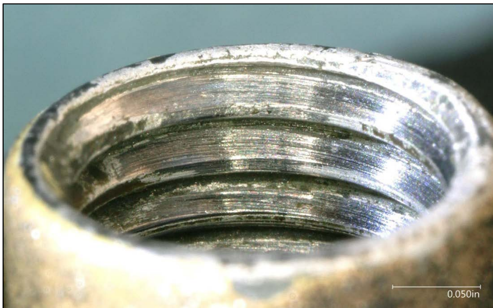
Figure 9. Optical image of the lower right nut plate after disassembly from the tail boom and after cleaning showing intact screw threads.
