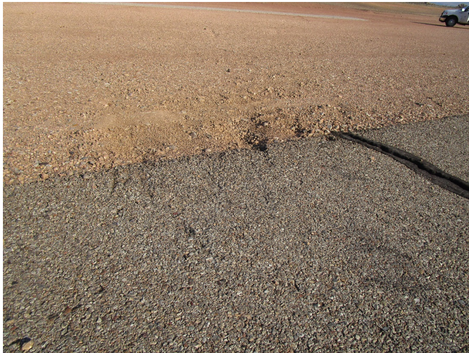
Figure 2: Damage to Runway Edge
