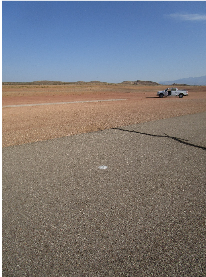
Figure 1: Damage to Runway and Adjacent Dirt
