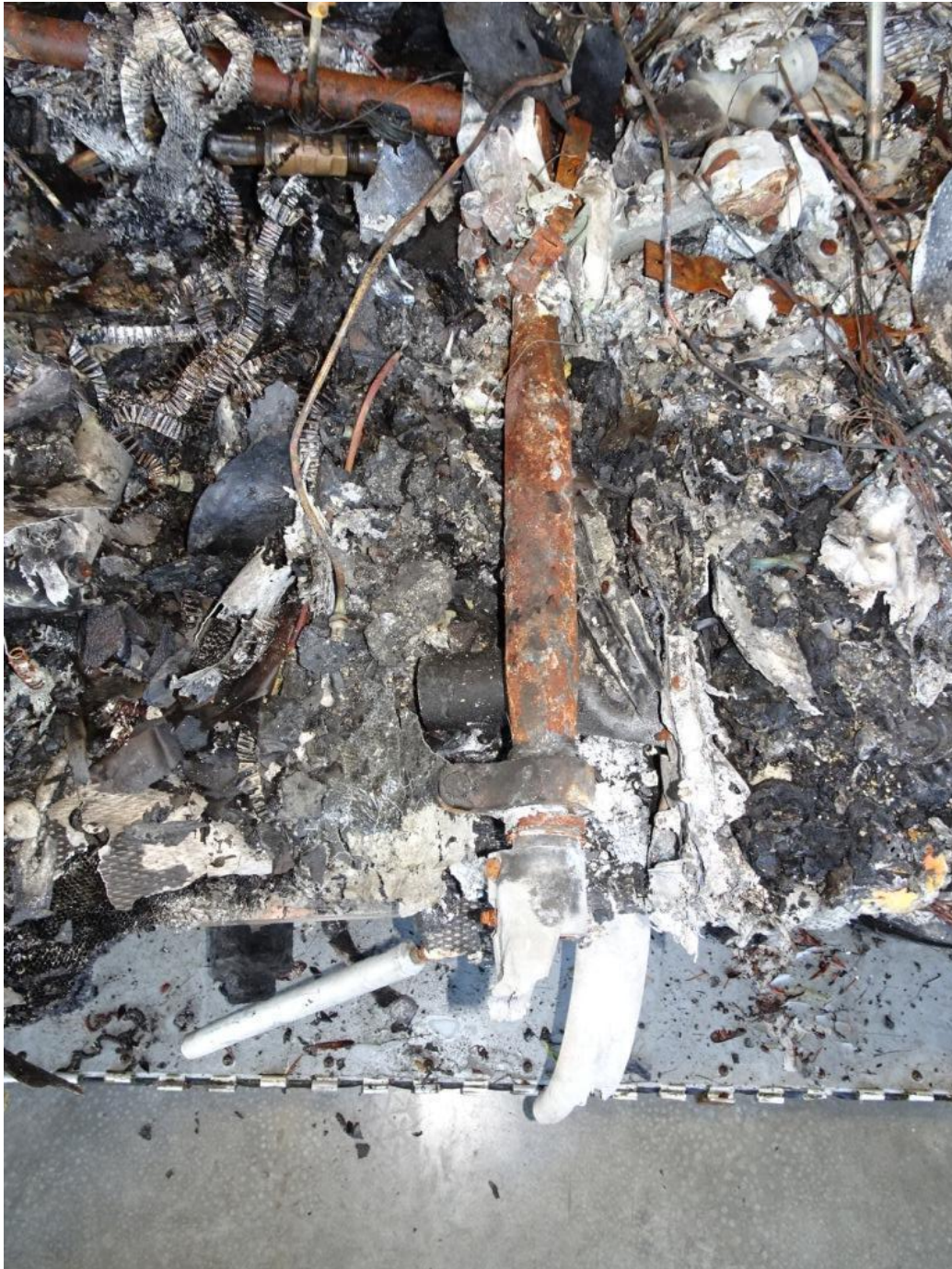
Figure 13 – Collective Jackshaft (looking right)
