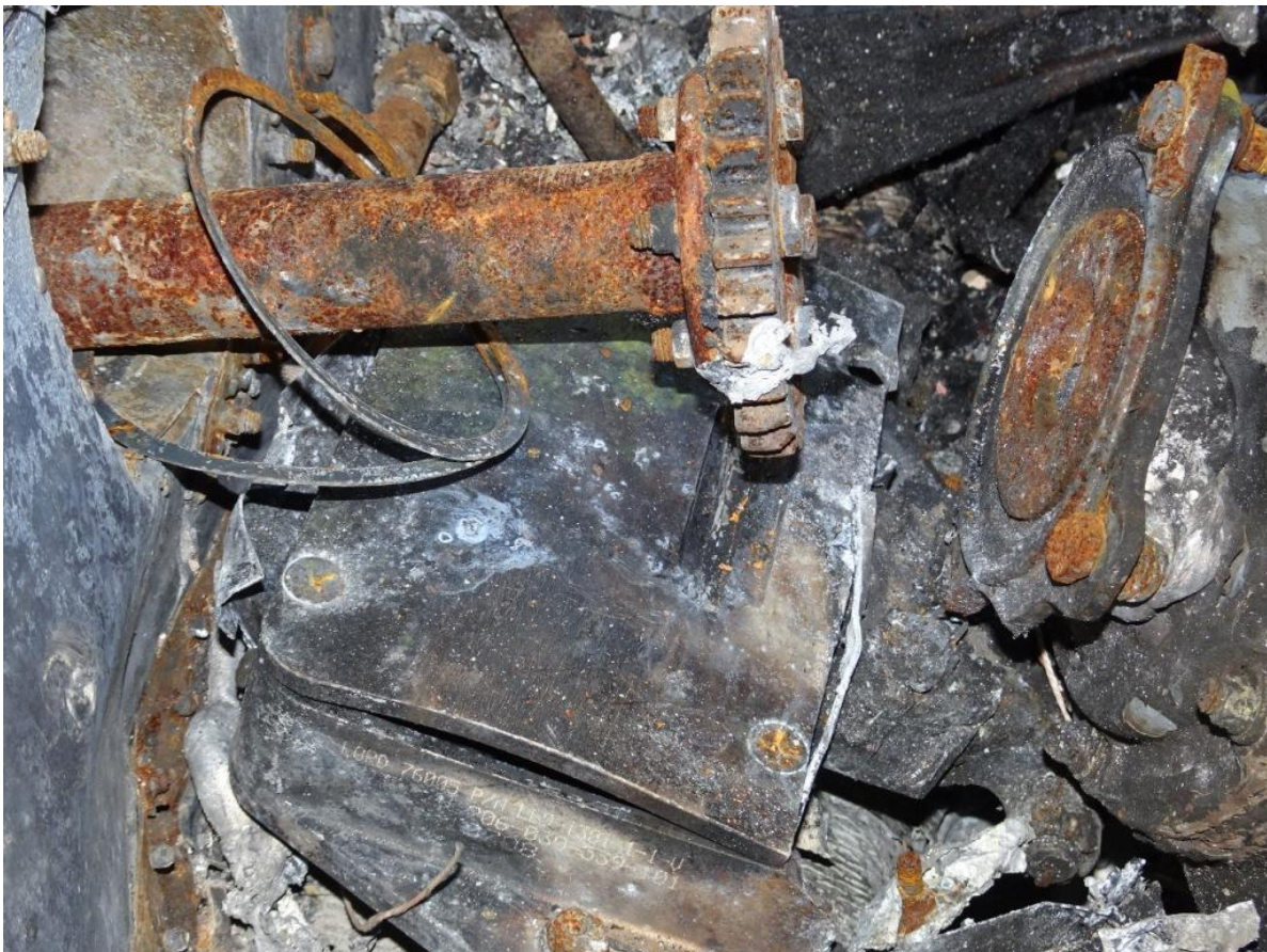
Figure 20 - Grinding-Damaged Isolation Mount
