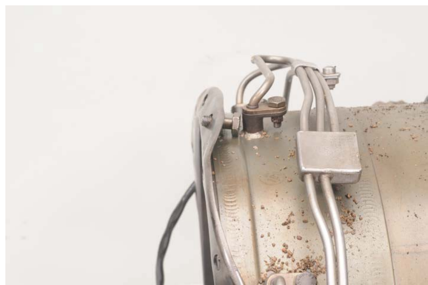
Figure 167. Engine Exhaust Duct
