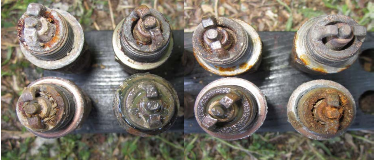
Figure 6 – view of upper and lower spark plugs
