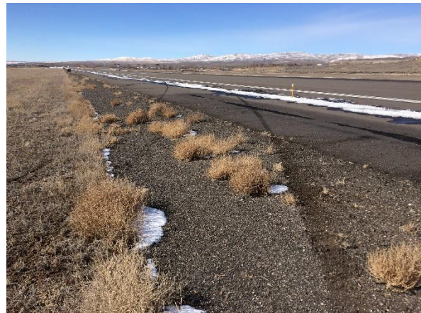
Tire marks and ruts. Facing west towards the approach of Runway 6 opposite direction of landing
