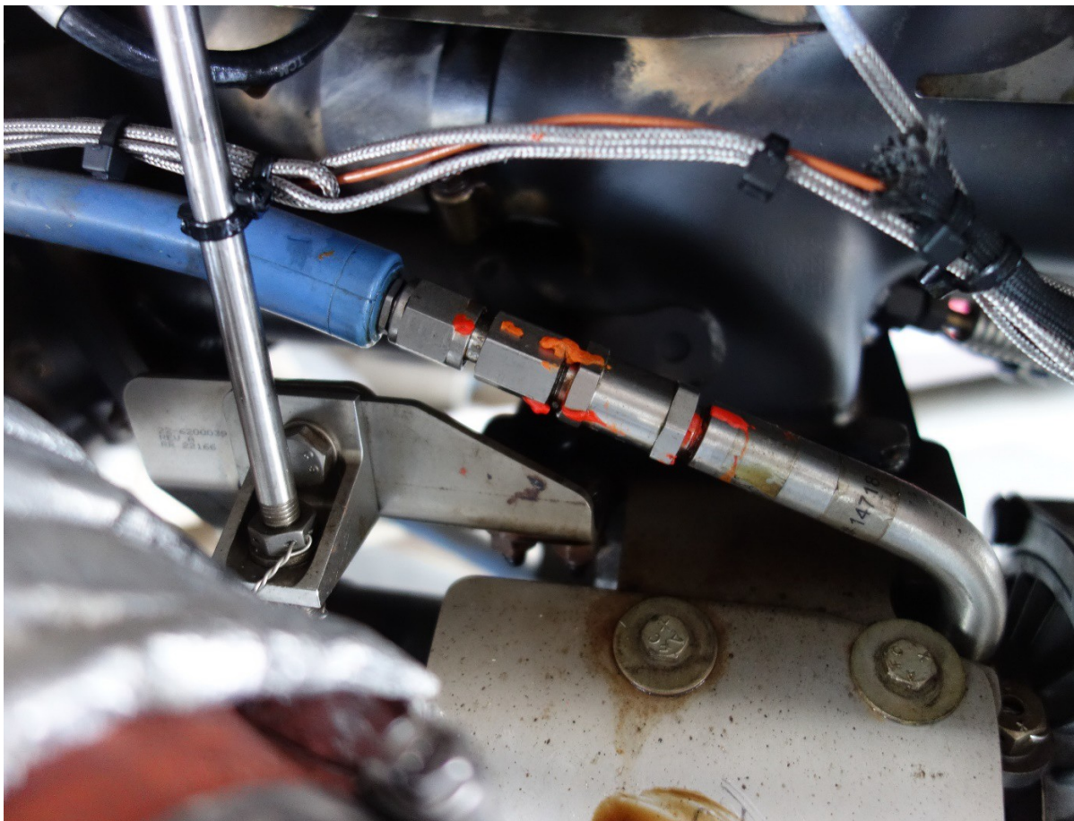
Figure 2: Loose b-nut fitting (right side).
