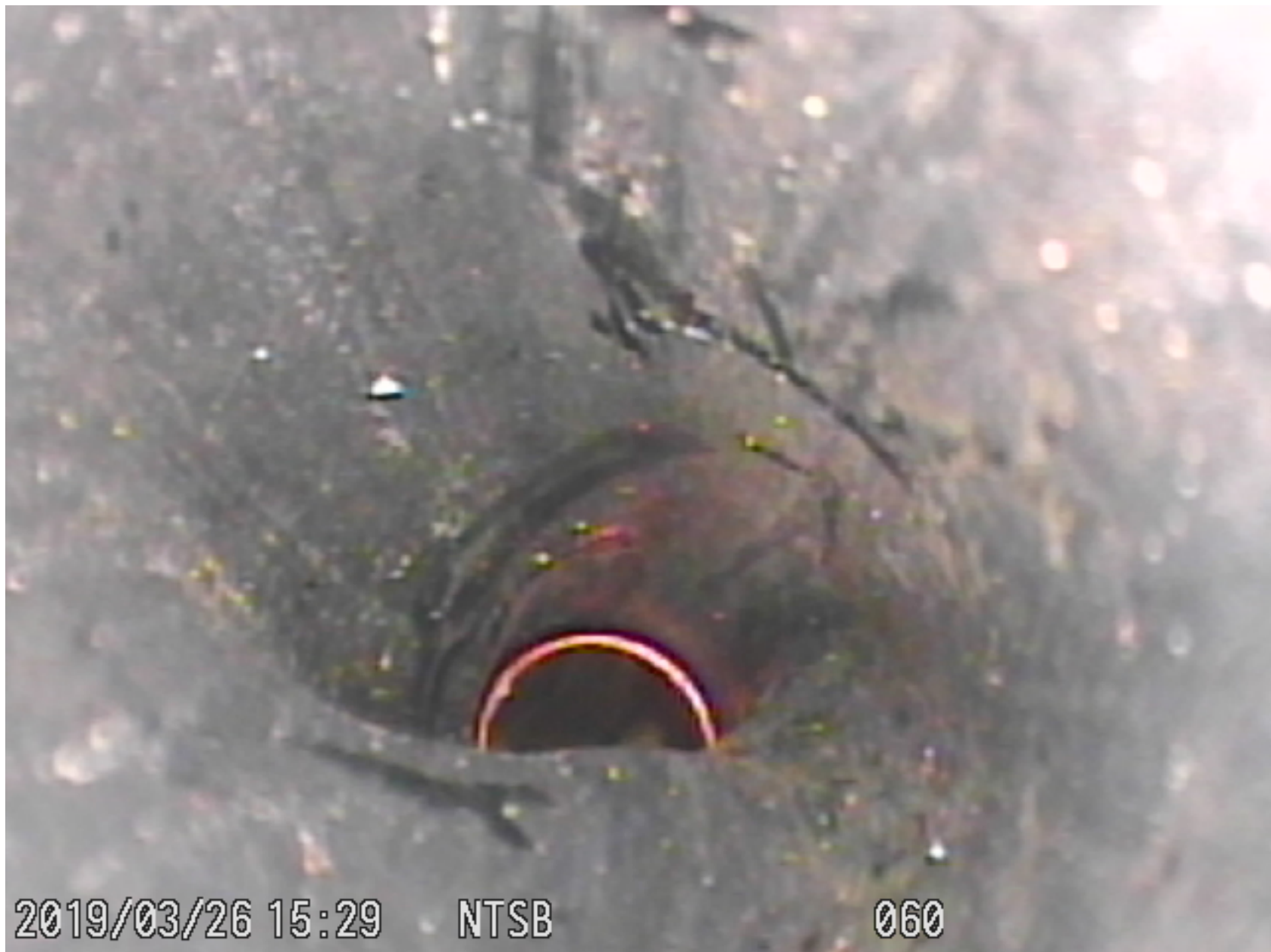
Photo 1 – Fuel Hose Inner Diameter View
