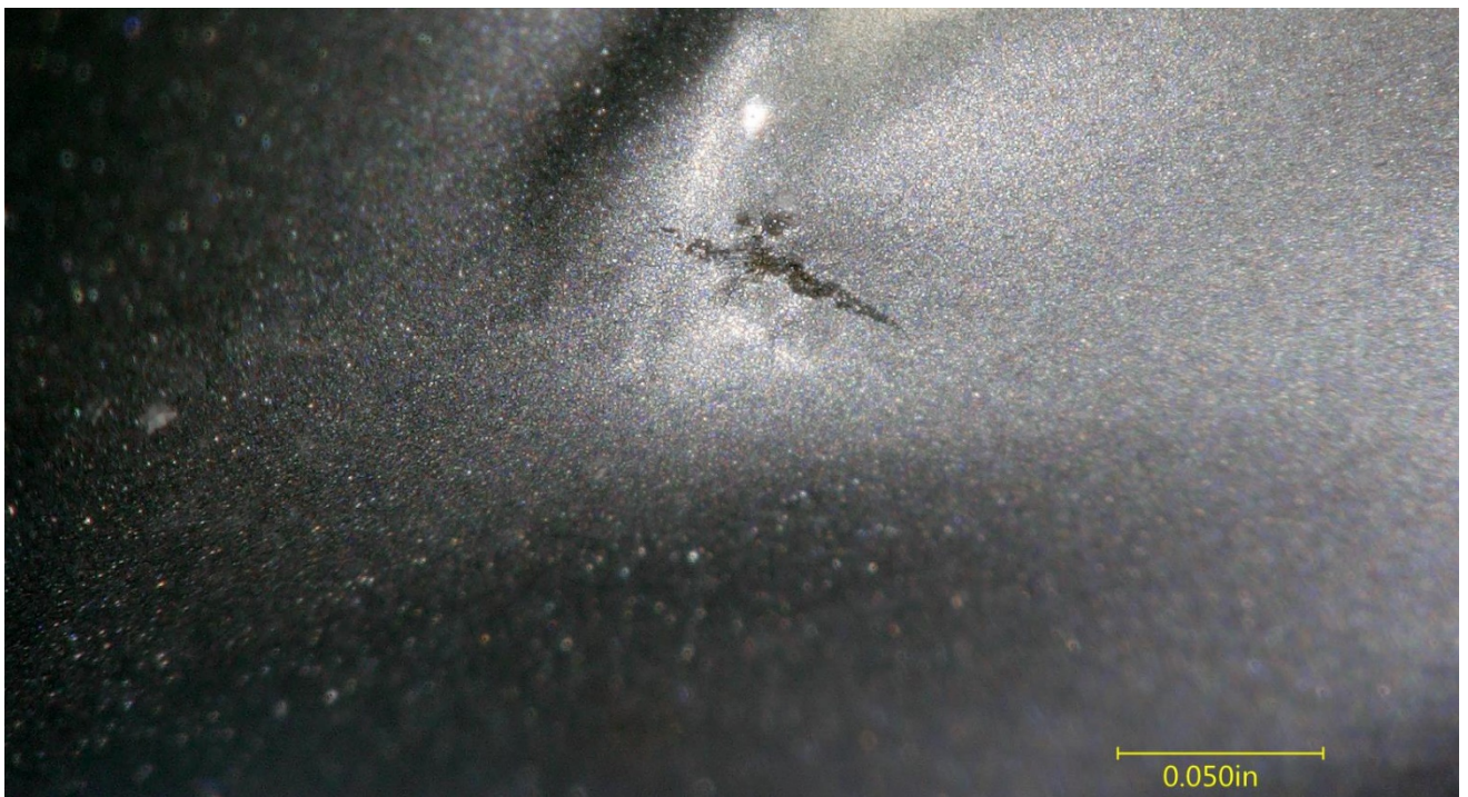
Figure 22 – Closer view of a surface crack on the intact tube joint.
