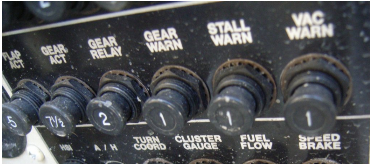
Figure 1 - SWS Circuit Breaker
