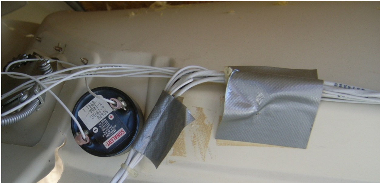
Figure 2 - SWS Horn (in situ)
