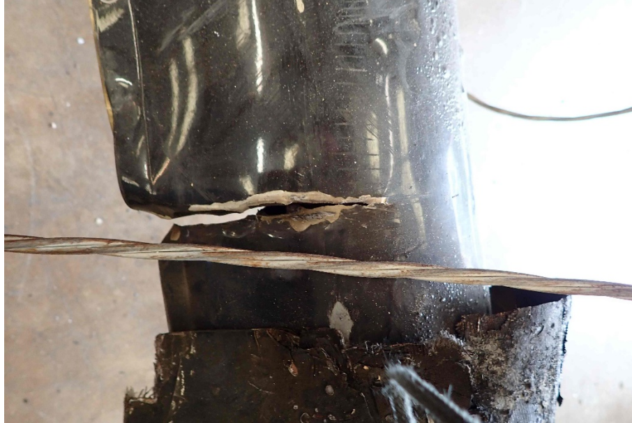
Photo 6 - Left Rear Strut Fairing and Cable
