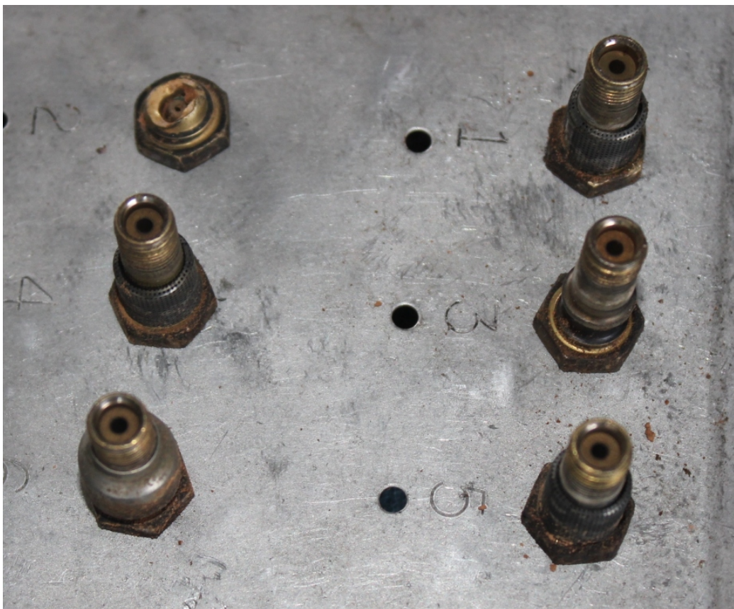
Figure 27 - Fuel Injection Nozzles
