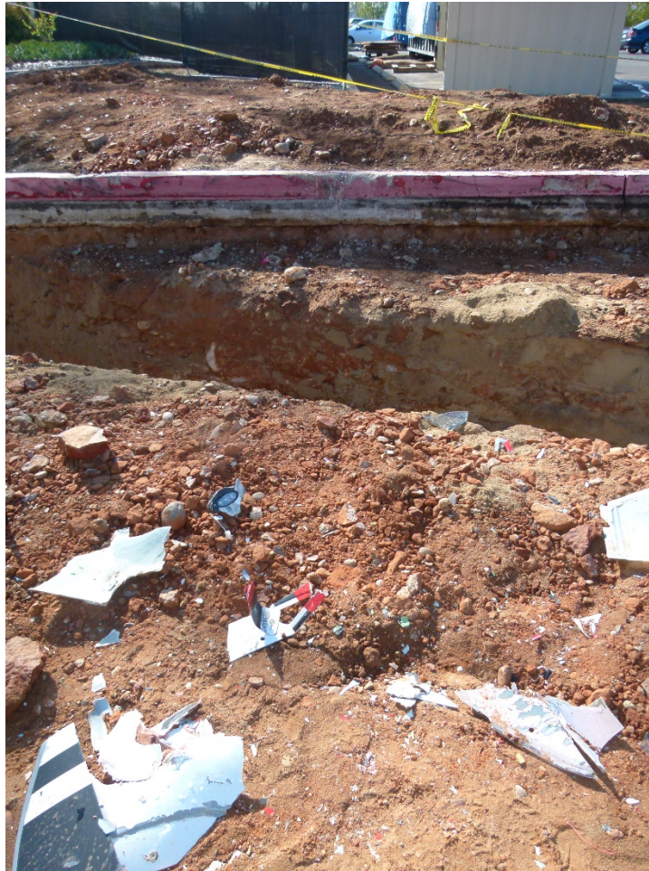
Figure 4: Impact Crater and Curb Damage from Left Wing
