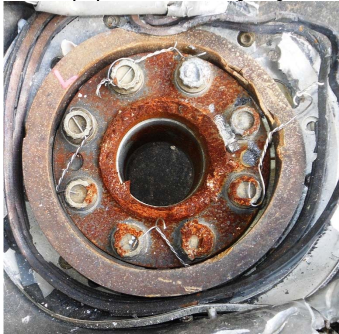
Photo #18 – Left propeller shaft mounting flange and hardware
