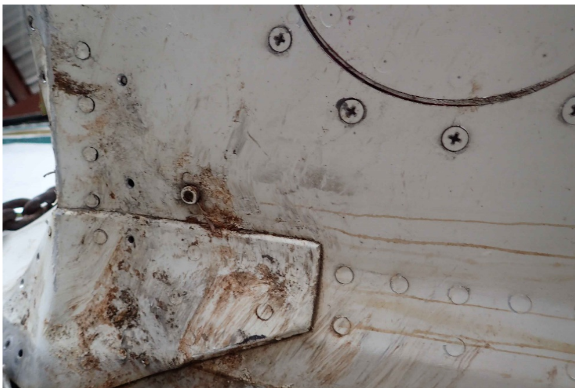
Photo 4 – Right Tank Sump Drain and Fluid Streaks
