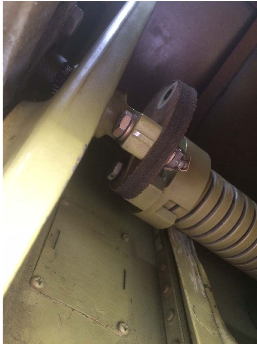
Photo 3 – Left Hand Varicam Drive Stop Coupling and AN174H7A Bolt (Courtesy of Neptune Aviation)
