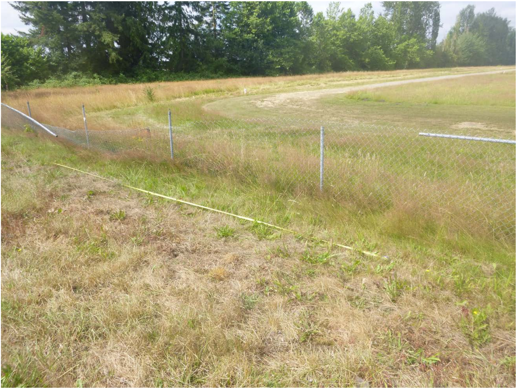
Photo 11 - Missing portion of the fence
