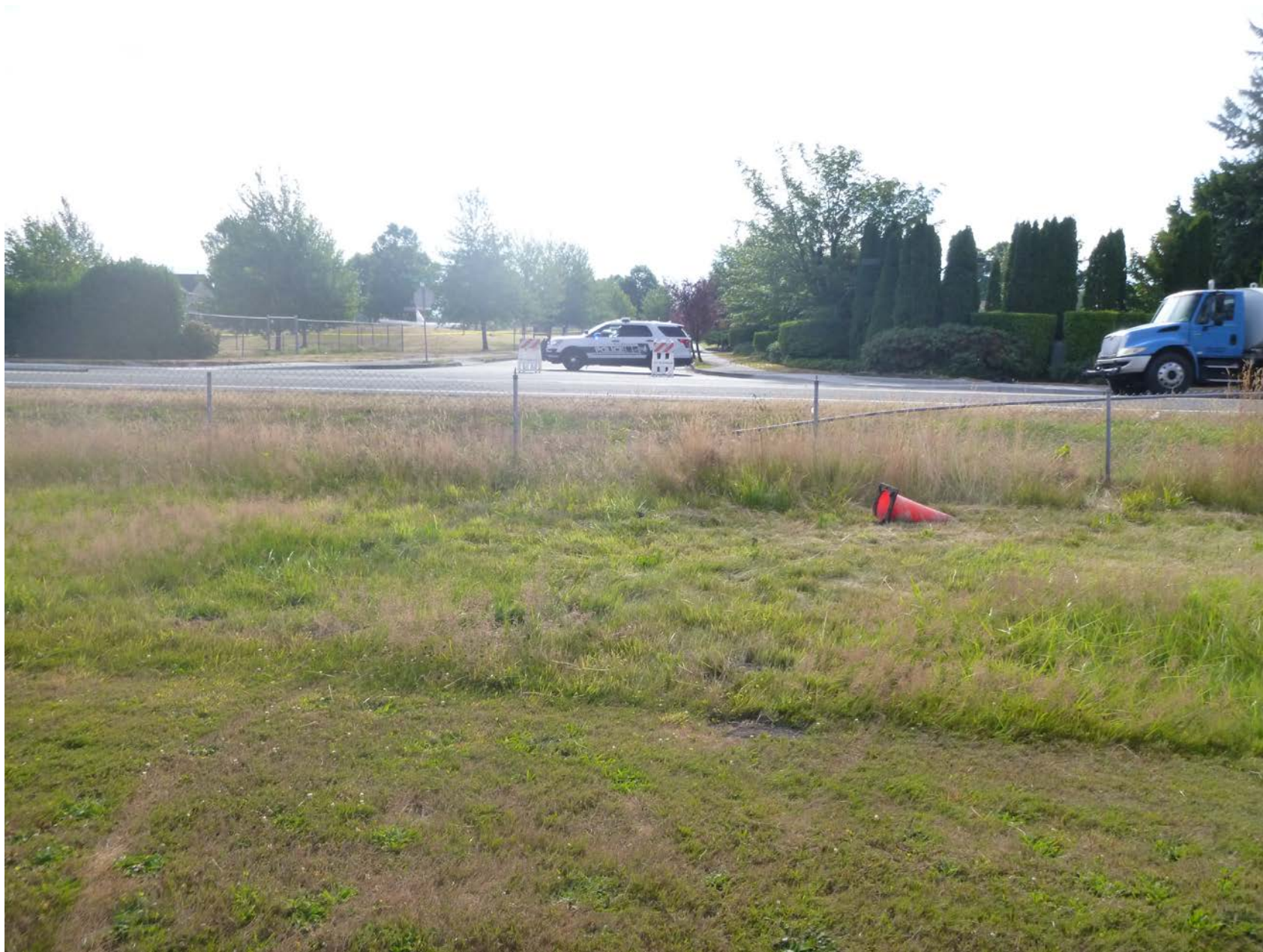
Photo 10 – Missing portion of the fence
