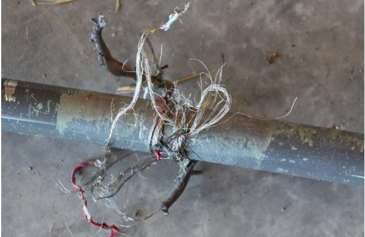
Figure 8 – Strobe Wire Wrapped Around Circumference of Drive Shaft
