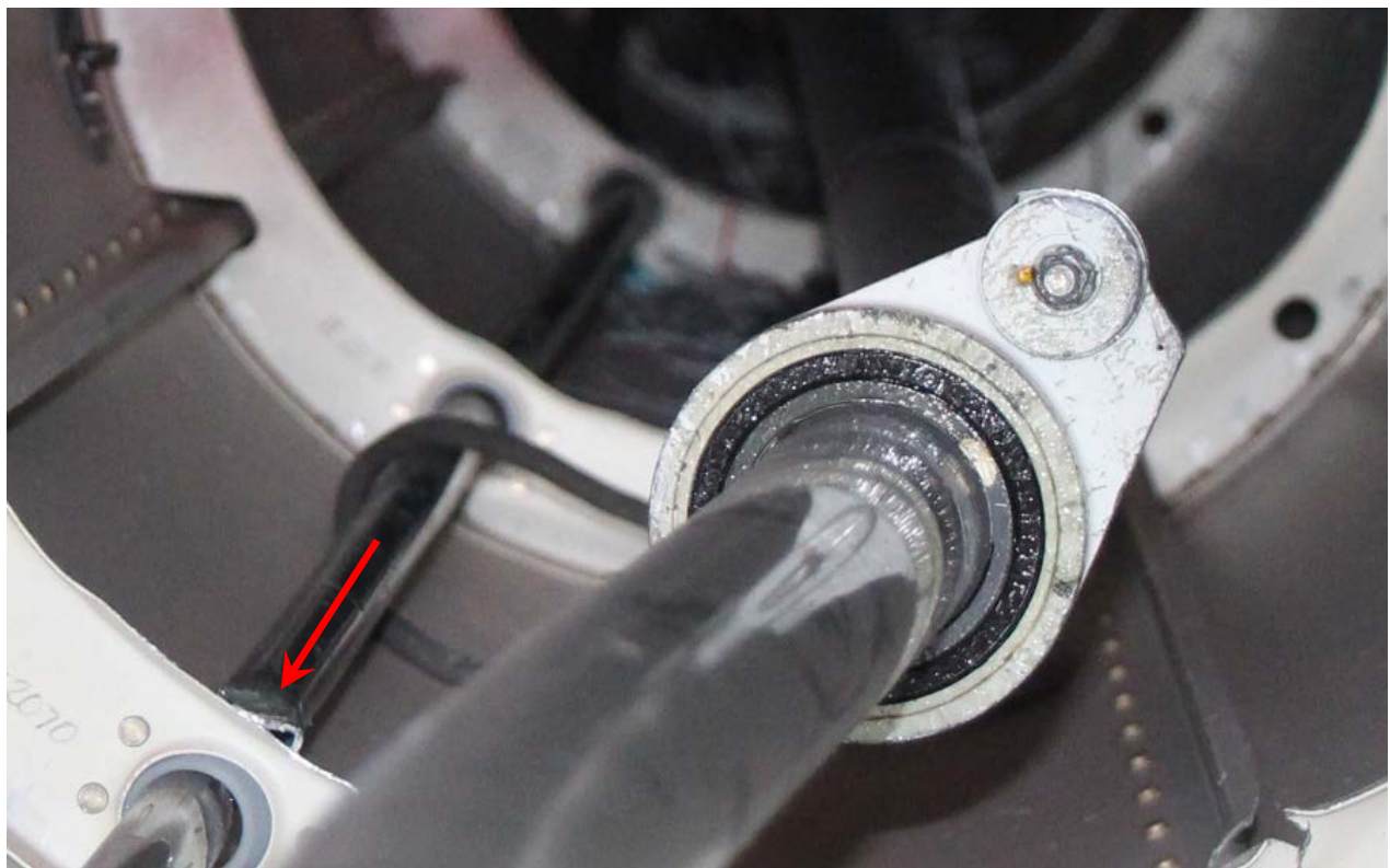
Figure 1 – Damper Bearing Secured to Bent Drive Shaft Without Hangar Bracket (red arrow shows severed -17 push/pull tube)
