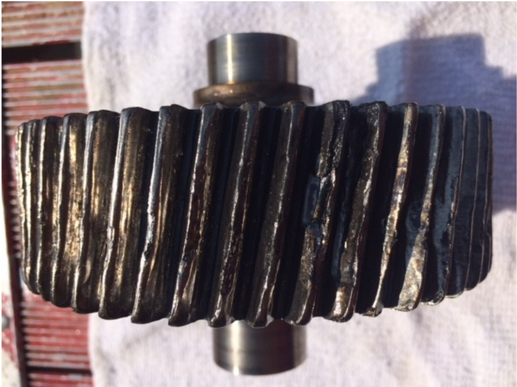
Photo 3 - Gearbox Idler Gear
