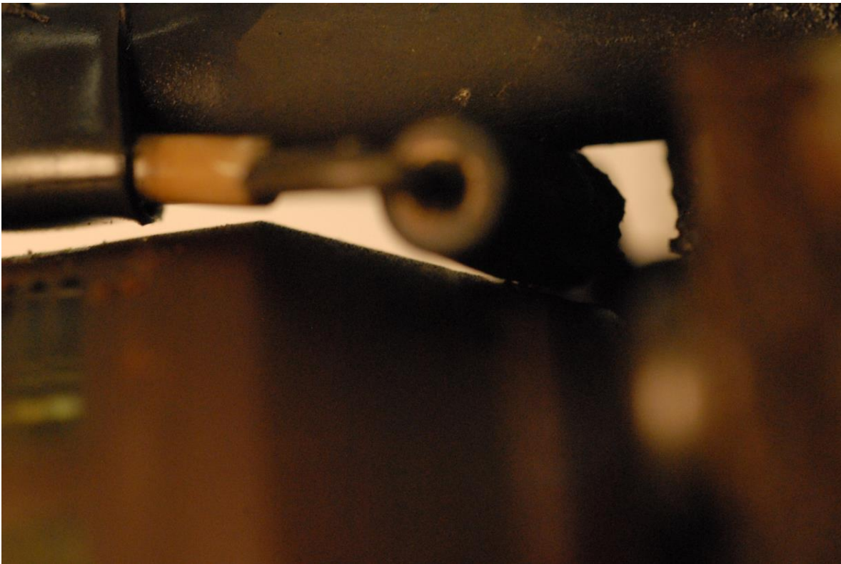
2C27-1 4H234 31Aug17_054 – Armature Contacting Thermal Fuse
