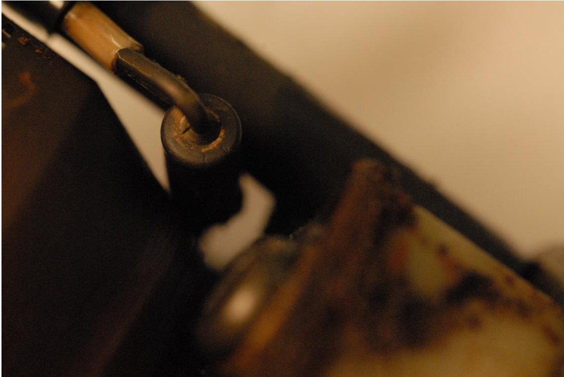
2C27-1 4H234 31Aug17_057 – Armature Contacting Thermal Fuse
