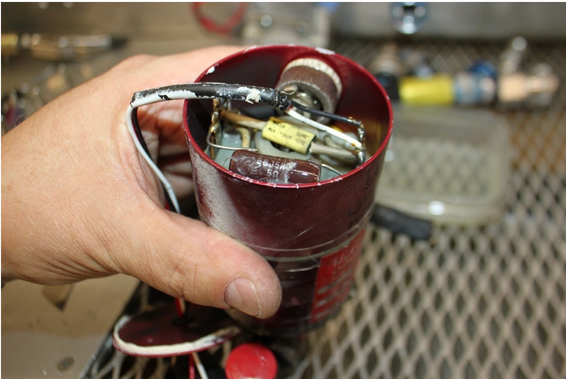
Figure 6: View of the Installed Resistor. Note the Markings.
