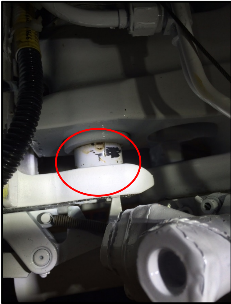
Figure 1: View of incident airplane's nose gear down-lock actuator piston (note white paint) as provided by the operator.
